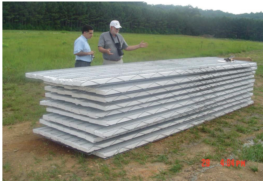
Figure 3 — Storage of SCIP system on the job site.
